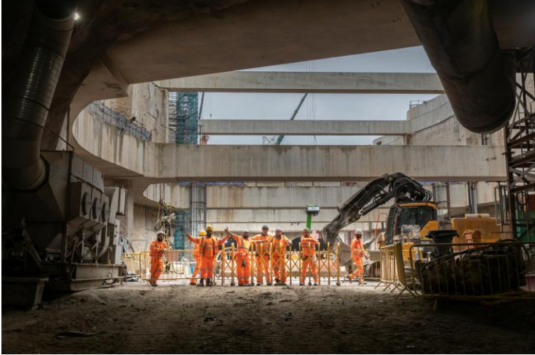
Inside the Victoria Road Crossover Box
