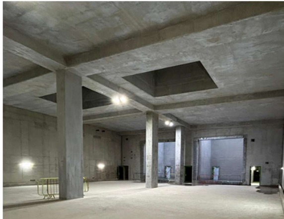
An example of a basement in one of the Chiltern tunnel ventilation shafts, ready for mechanical and electrical outfitting in 2026
