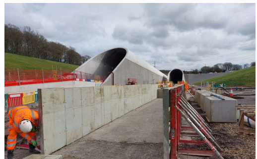
An Align worker puts the finishing touches to the concrete walkway at the north portal in March 2026.
