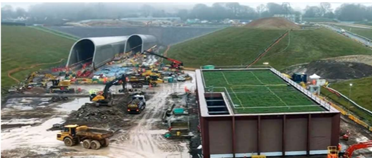
A view of the Chiltern tunnel north portal and ancillary building, looking toward Frith Hill, from February 2026.
