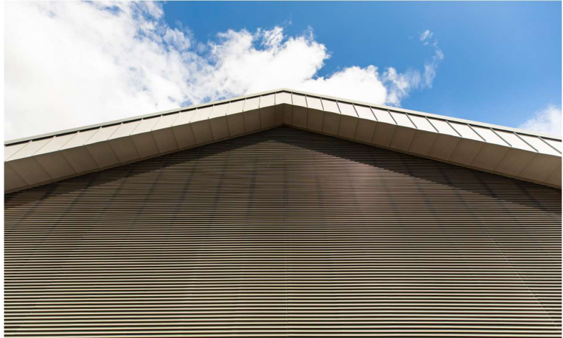
The pitched roof of the main building at the Chalfont St Peter site.
