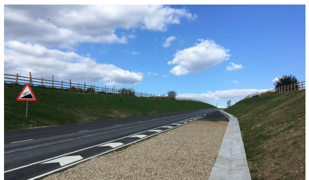
The temporary access road linking the Chalfont St Peter construction site to the A413 Amersham Road will be removed this year.
