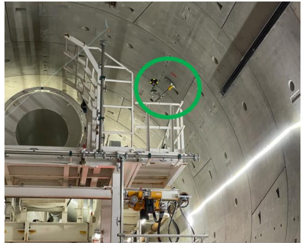
Above: Survey Control Marker Prism high above the last TBM gantry on the tunnel wall for measuring angles and distances for the TBM guidance system.
