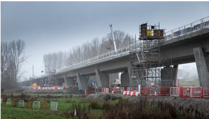
We have now completed 60% of the poured concrete deck at Edgcote viaduct.
