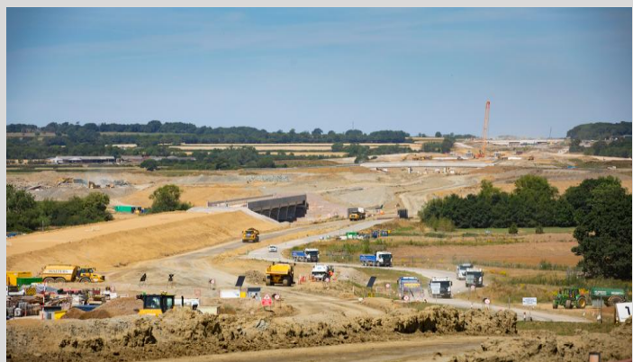
At Highfurlong Brook, the earthworks team worked throughout 2025 to grade and stockpile earth.
