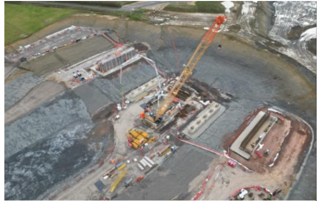
Foundation piling at Stoneton Lane green bridge, has been completed ahead of building the main structure.
