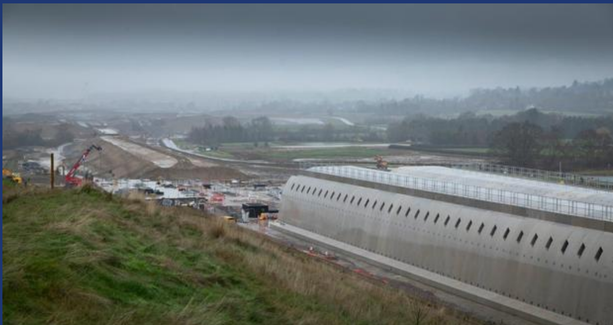
The portal pieces at the northern end of Chipping Warden green tunnel and the earthworks towards Highfurlong Brook viaduct are progressing.
