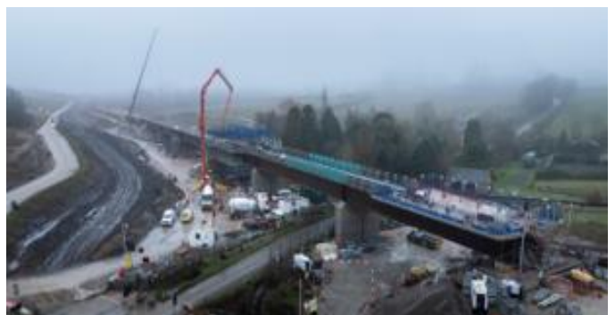
At Lower Thorpe viaduct, the traveller is positioned above the structure, while concrete is being delivered to the deck using a crane-mounted pump.
