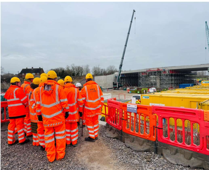
The image above shows Winslow Lions admiring the progress of School Hill overbridge in Calvert and receiving an update from the site manager.
