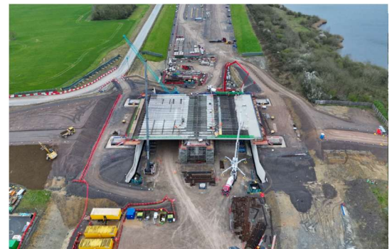
School Hill overbridge with Jubilee lake and Calvert Green village to the right.
