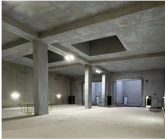
An example of a basement in one of the Chiltern tunnel ventilation shafts, ready for mechanical and electrical outfitting in 2026
