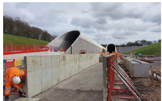
An Align worker puts the finishing touches to the concrete walkway at the north portal in March 2026.
